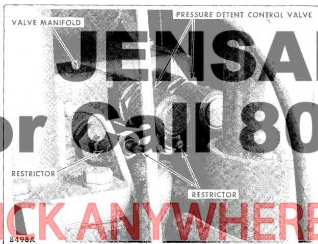
Fig. 15 Remote Valve Manifold and Valve Restrictors
