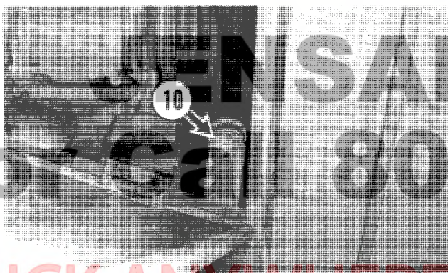
Key disconnect switch (10).
