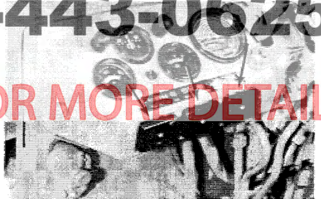
Figure 24: Electrical Fuse Boxes
